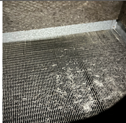
10. Corroded heating water coil
