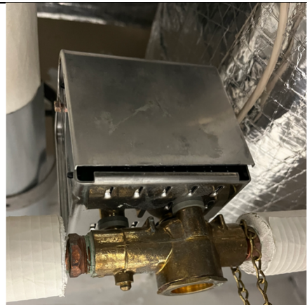
4. Typical control valve from 1999
