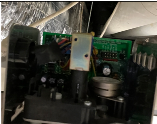
5. Cover removed off 1999 control valve.
