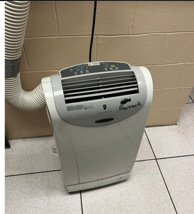
8. Supplemental cooling observed in dispatch
